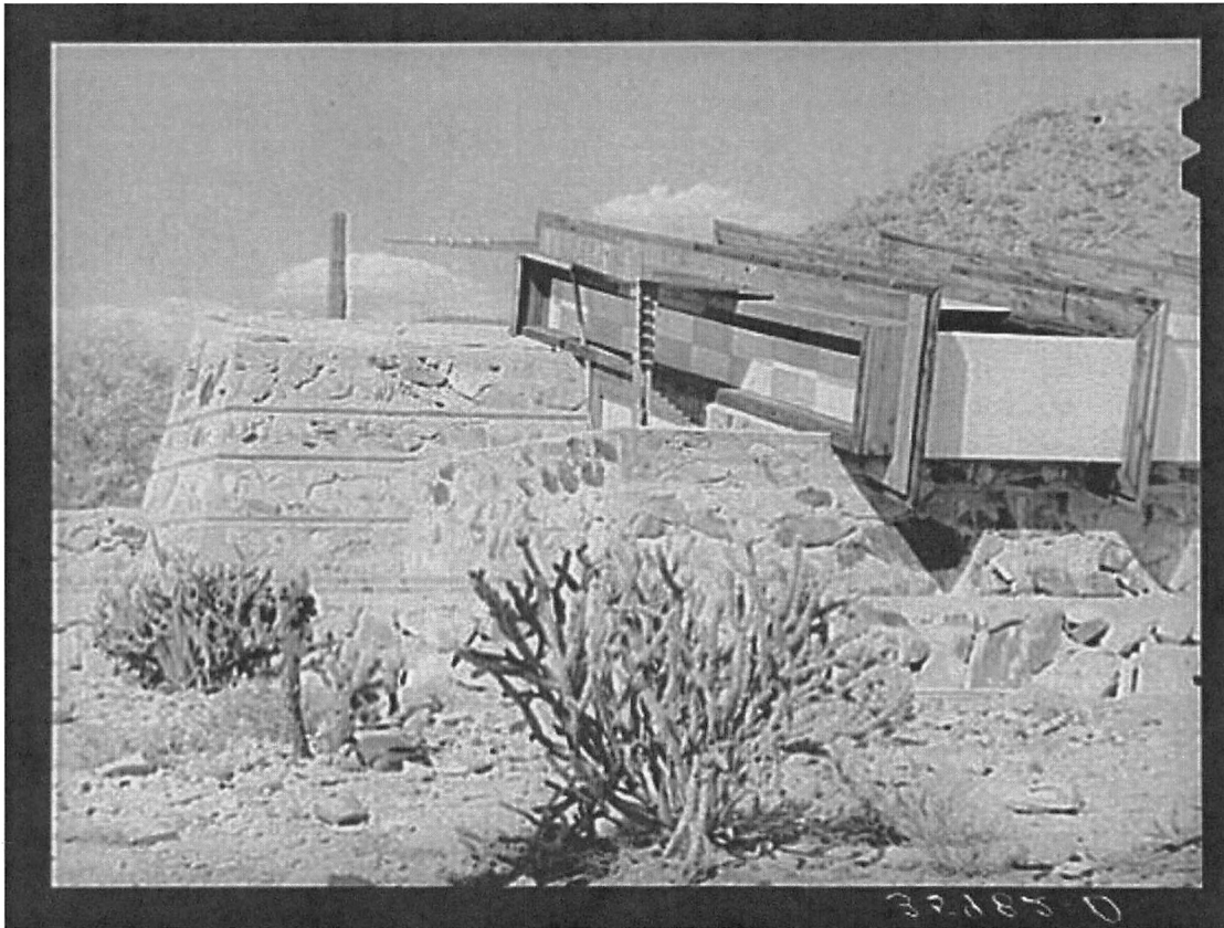
Detail of construction of Frank Lloyd Wright's winter quarters at foot of McDowell Mountain. Maricopa County. Arizona.
